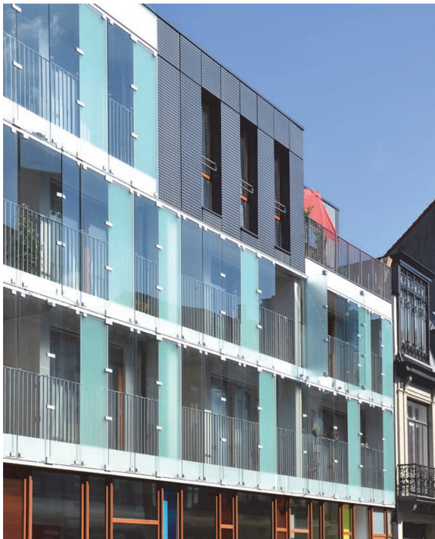
Fig. 1.1 – The building envelope is often designed to increase passive solar gains during winter, however this may create overheating during summer if not adequately controlled.
